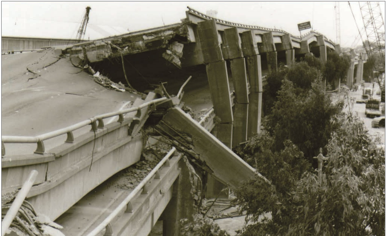
FIGURE 7: Collapsed Section of the Cypress Street Viaduct
