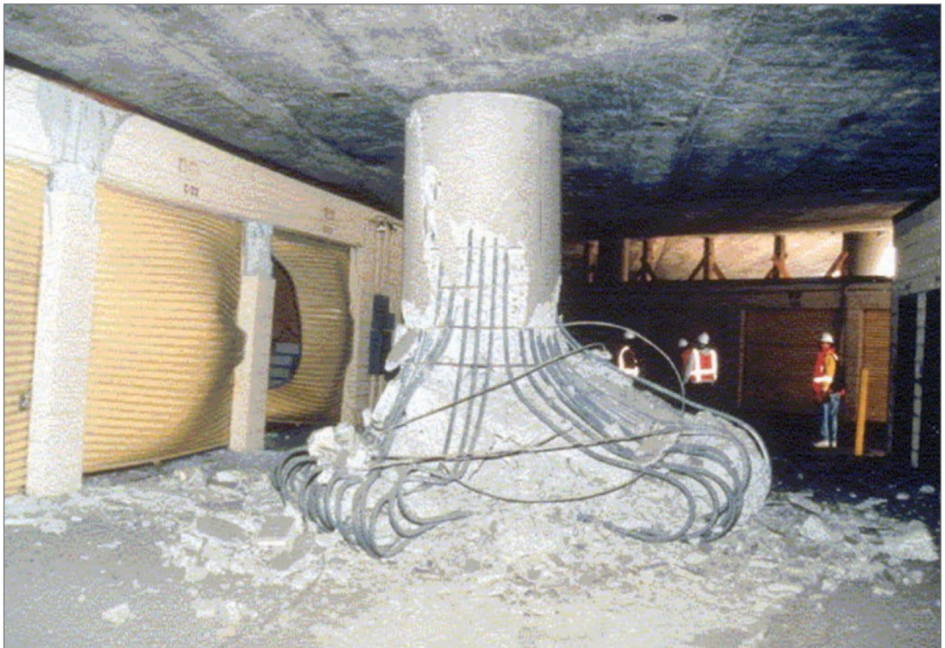
FIGURE 9: Failure of the Santa Monica Viaduct Column
