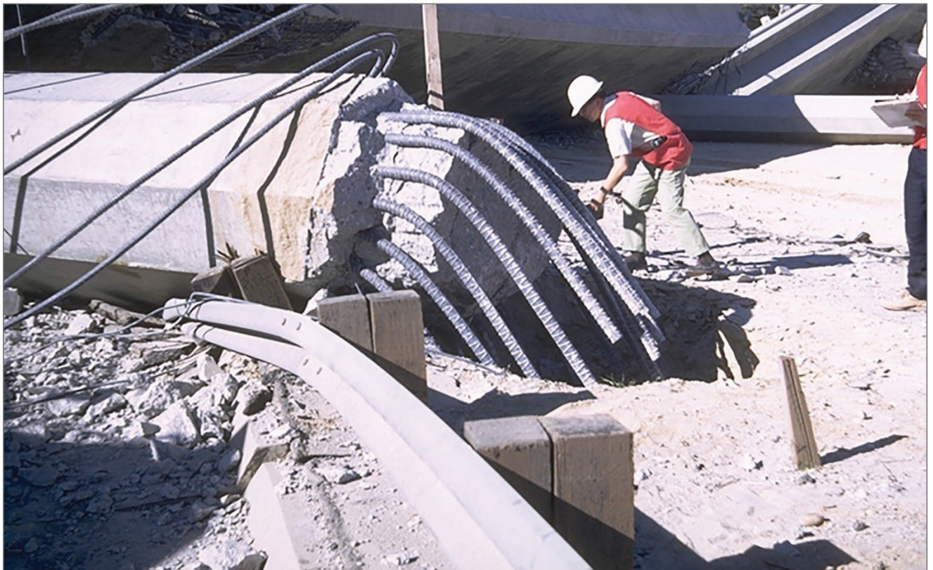
FIGURE 4: Lap Splices at the Column Base Caused Collapse at Route I-210/I-5 Separation and Overhead
