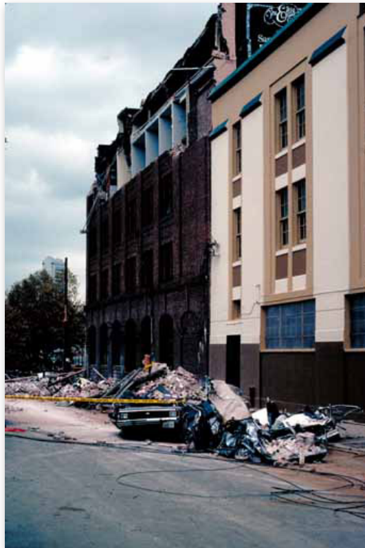
Earthquake shaking caused the unreinforced brick parapet and façade of this building to collapse, killing people on the ground.
