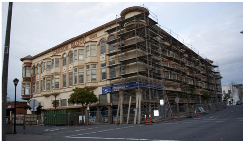
This retrofit project in Eureka took over 25 years to complete. It relied on federal tax credits for historical buildings and a loan from the city’s Community Development Block Grant.
