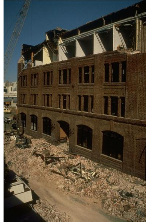
Collapse of inadequately retrofitted brick building onto cars in San Francisco after the 1989 Loma Prieta earthquake.
