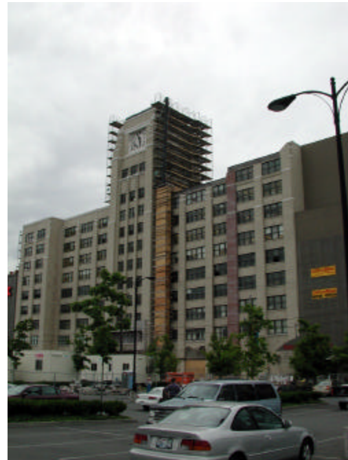
Figure 4 Starbuck's Corporate Headquarters Under Repair, Seattle, WA
