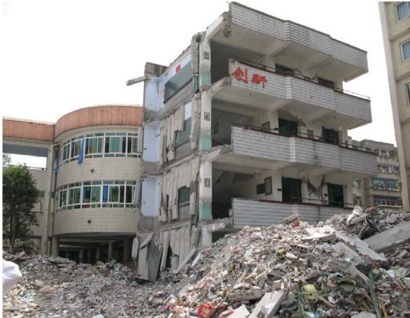
Figure 2: Damage to Elementary School in Xing Fu Township, Dujiangyan, during the 2008 Magnitude 8 Wenchuan Earthquake in China (Photo Credit: Miyamoto International)
