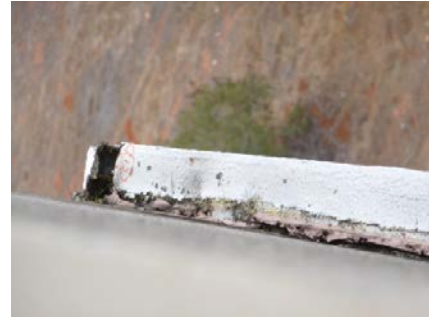
Fig. 2(c) Gap between exterior CFS framed wall system created due to ground motion and soot from smoke
