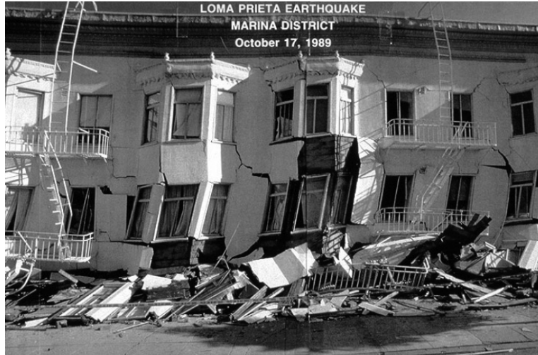
Figure 2 Marina District Apartment building damage during the 6.9 magnitude 1989 Loma Prieta earthquake. Two nearby public schools were not damaged and were used as emergency shelters.
